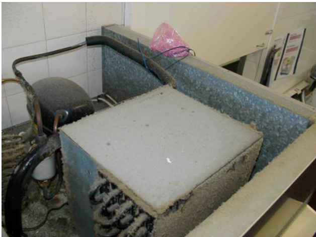
Condenser unit prior to cleaning
